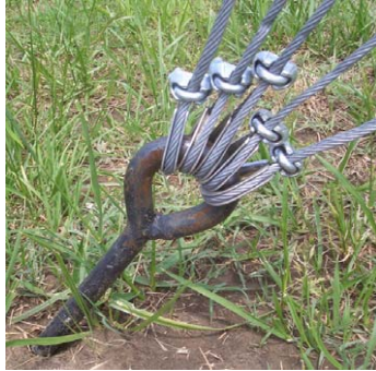
Figure 5: Tower guy wire attachment to anchors
